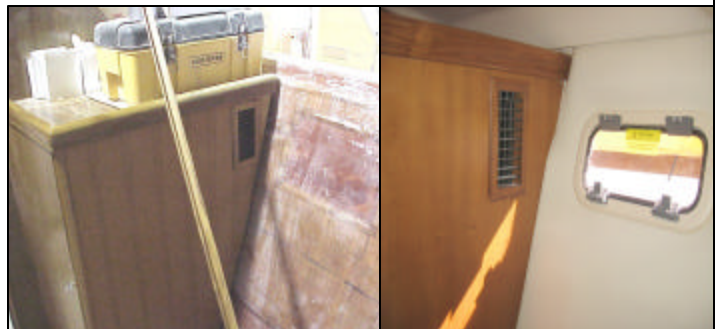
QB starboard side hanging locker AC grill complete, re-install cedar panel back inside hanging locker
