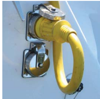
Fig. 8.5 the stainless shore power connector located on transom port side next to mooring cleat. the upper connector is for AC connection, and the lower connector is for TV antenna connection.
