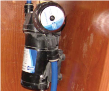
Fig. 9.3. Replace the strainer periodically for better performance of the entire fresh water system. The water pump unit with strainer locates underneath the galley shelf.
