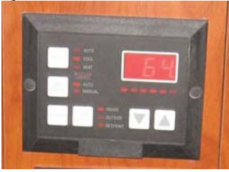
Fig. 8.4 shows one of three air conditioning unit wired remote control panels. For more detail information, please refer to the A/C owner's manual
