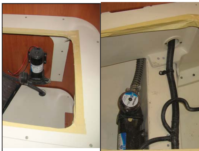
Fig. 10.3 (Forward and Aft Shower Sump Pump)
