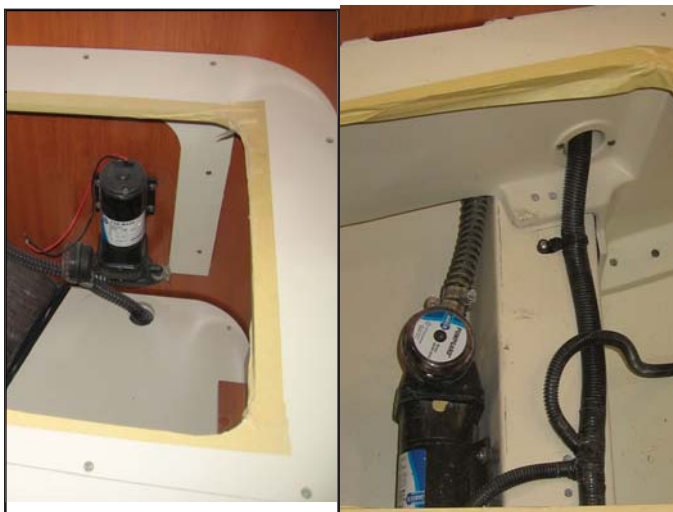
Fig. 10.3 (Forward and Aft Shower Sump Pump)
