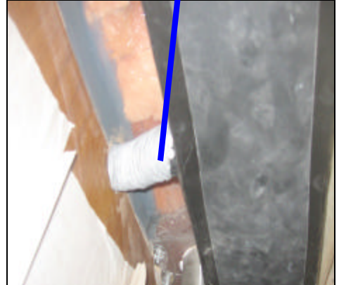
2" air duct goes to fwd vanity
