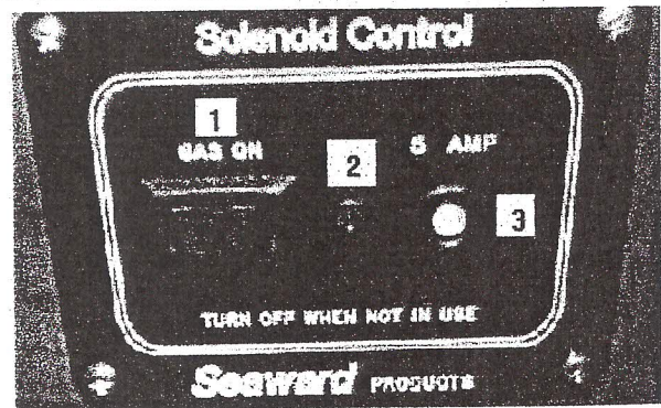
LP. GAS PANEL LOCATED AT GALLEY
