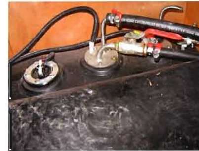
Supply valve Fuel
