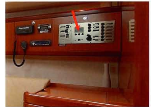
Gauge - Electrical panel
