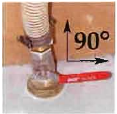
Thru-hull fitting closed
