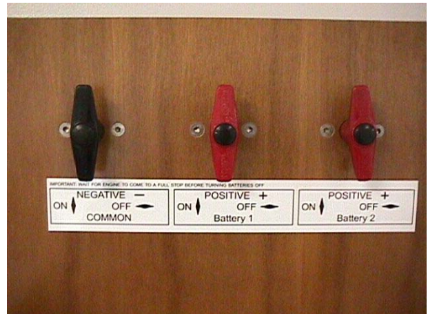
Everything is ON, 12VDC power available to start engine and/or run equipment
