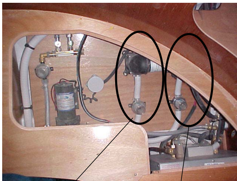
PUMP STATION UNDER STBD SETTE
